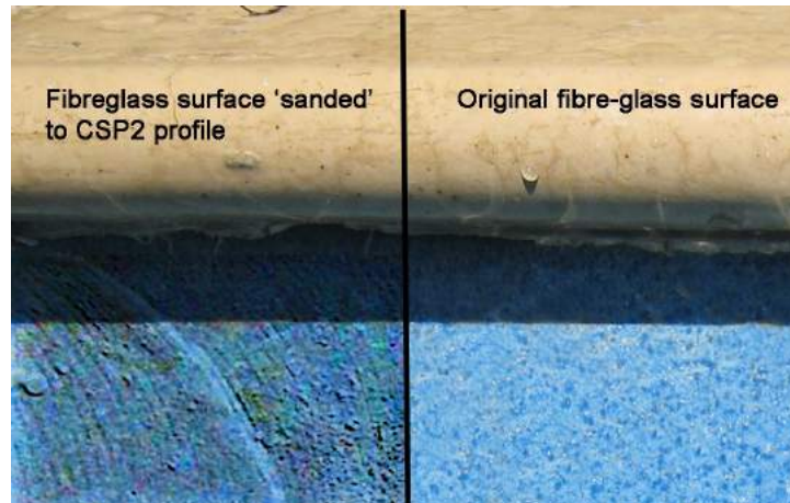
Figure 7. A schematic showing a fibre-glass pool that has been surface prepared to CSP2 profile.
