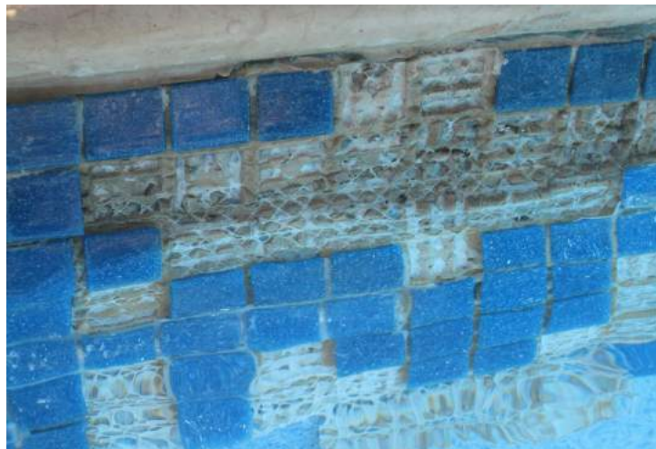
Figure 8. An example of mesh mosaic tiles that have failed at the waterline because of an inappropriate adhesive choice for a fibre-glass pool shell, but also because the mesh adhesive was water softening and obstructed the adhesive contact coverage with the tile itself.
