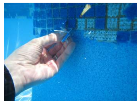
Figure 6. An example of a tiling installation where the pool shell has not been properly prepared prior to the application of 'waterline tiles'. The adhesive has not bonded.
